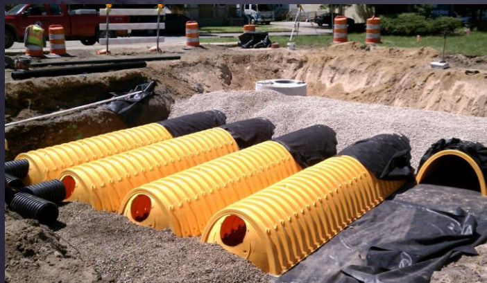
Figure 10: Underground Water Storage
